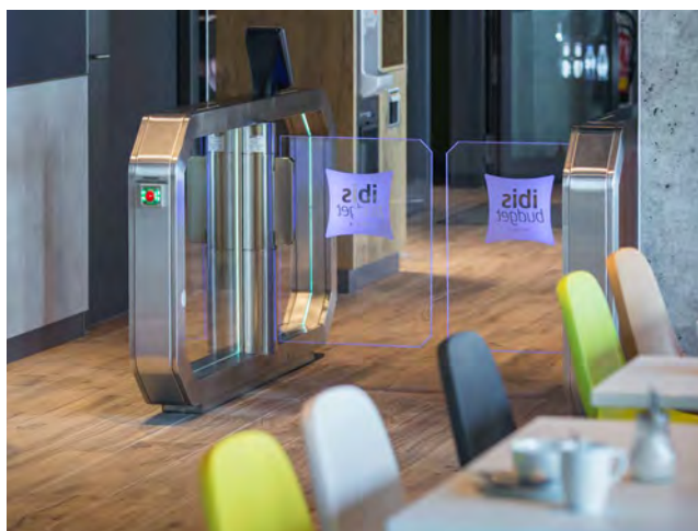
ACCESS CONTROL to the breakfast room
